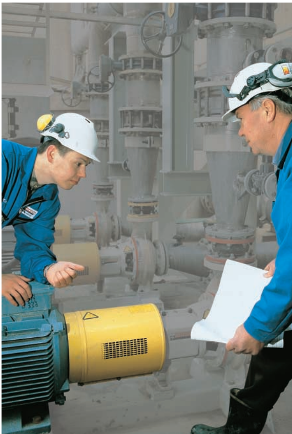
Two ABB ACS 600 AC drives - supplied and installed by ABB Drives Alliance partner EDC (Scotland) Ltd - keep the water flowing at the Helensburgh pumping station in West Dunbartonshire, saving West of Scotland Water £80,000 worth of energy
