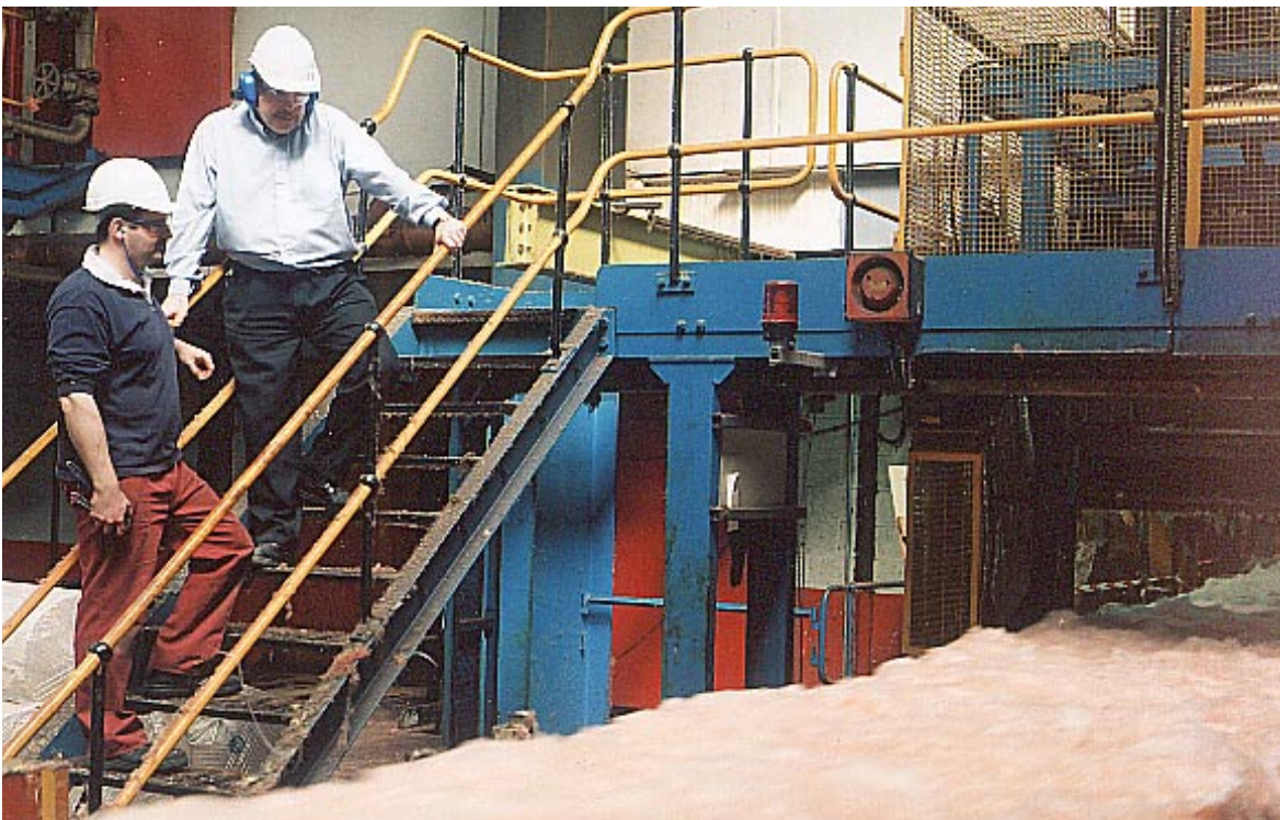
Insulation manufacturer KnaufAlcopor is saving £50,000 in energy per year since installing ABB AC drives from Drives Alliance Partner Central Electrical
