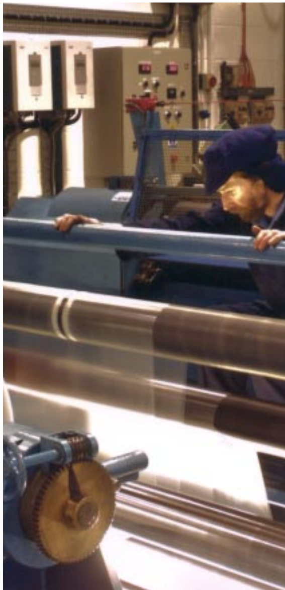
BPI Films is saving 66% costs on a slitter-rewinder machine following the installation of ABB variable speed drives
