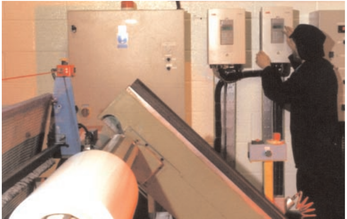
The ABB ACS 600 drives have reduced the demand of the principal motor
